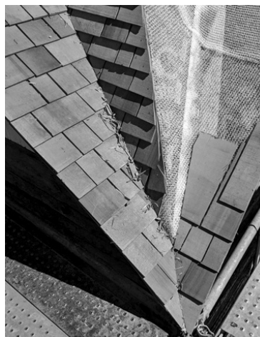
Corner detail showing yellow Cedar Breather product laid over Ice and Water Shield, providing an air barrier underneath the new cedar shingles. (May 20, 2019, photo courtesy NPS)
