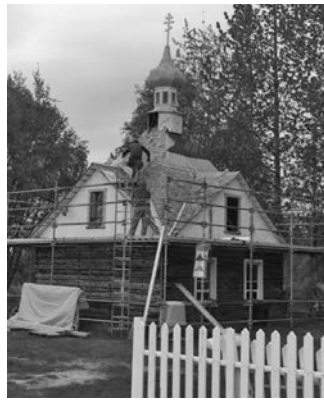
Al Williams and Doug Buttery completing upper portion of shingle work. (May 25, 2019, photo courtesy Dorothy Gray)
