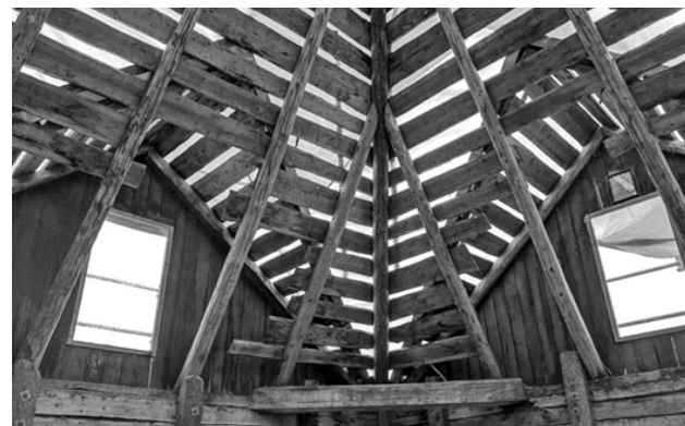
View looking up at the roof rafters and exposed sheathing after shakes have been removed and temporary plastic sheeting is being installed. (May 5, 2019, photo courtesy NPS)
