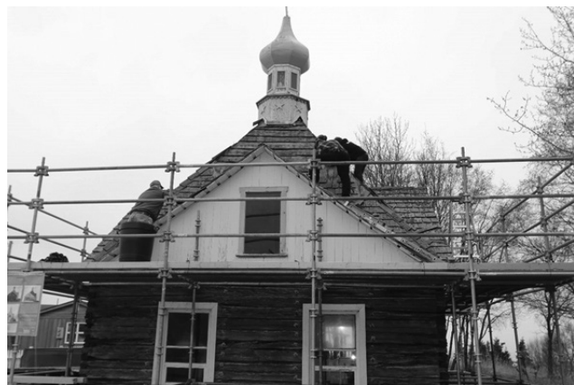
Church volunteers removing various portions of the old roof. (May 5, 2019, photo courtesy NPS)
